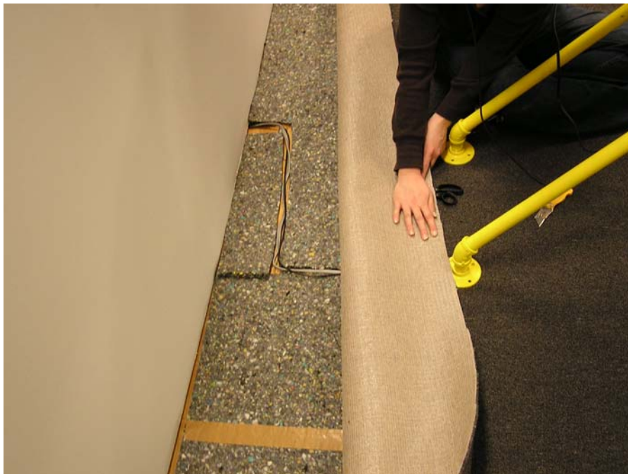
Educational Development, 2007. Solution for wires to come through pipes of SeeSaw and under carpeting and wall.
